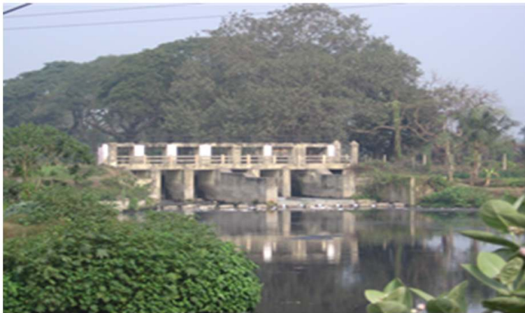
Fig. 4. Bantala Lock Gate, originally used to supply wastewater to stabilisation ponds without pumping
