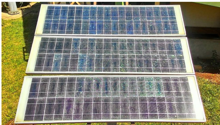
Figure 1. Photovoltaic system used in power supply
